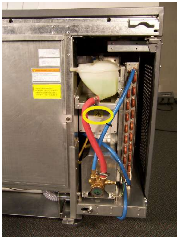
Figure 43: Location of a hazardous voltage label
